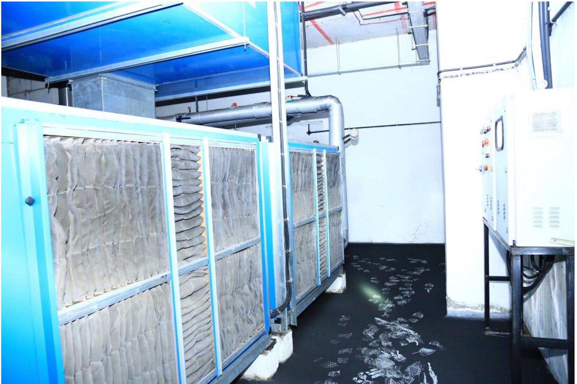
Failure of smoke detector to signal closure of HVAC fire damper seen as soot deposit on floor of AHU room after smoke entry. Notice soot on filters.
