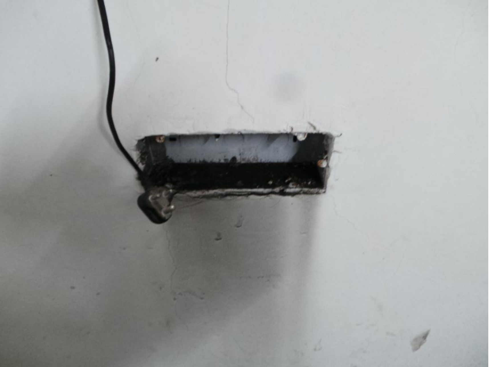
Compartmentation example: weakening of 2 hr rated enclosure showing signs of smoke ingress due to reduced wall thickness
