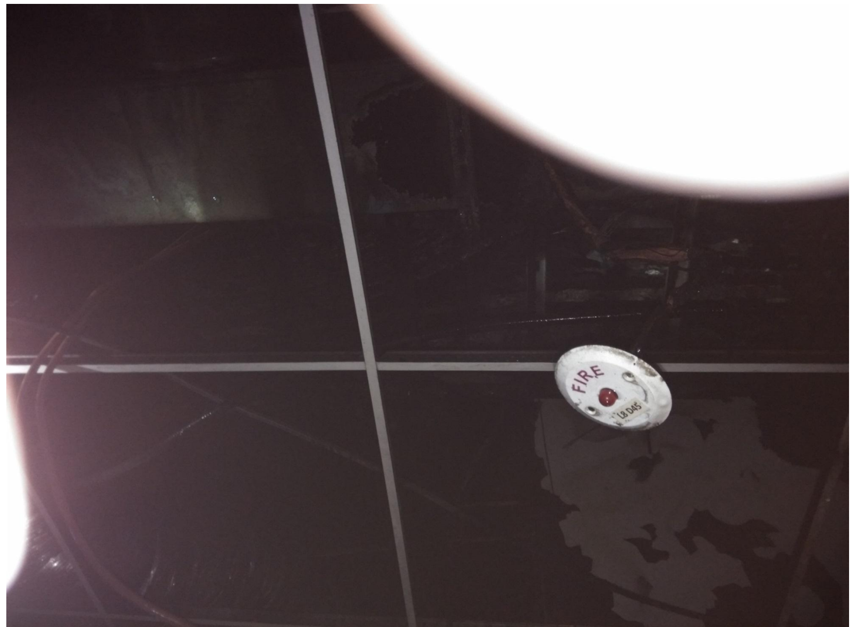
Response indicator with address of overceiling smoke detector seen after fire damage
