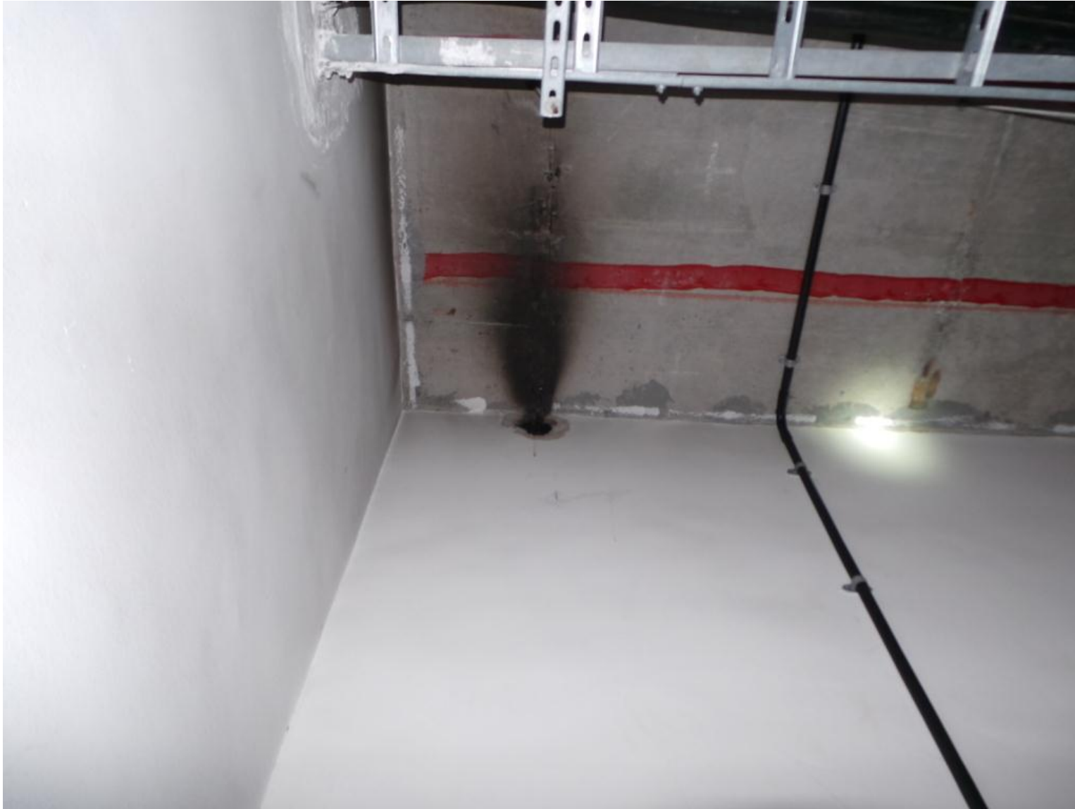
Compartmentation example: Unsealed post construction puncture in a 2 hr rated enclosure showing smoke ingress after fire
