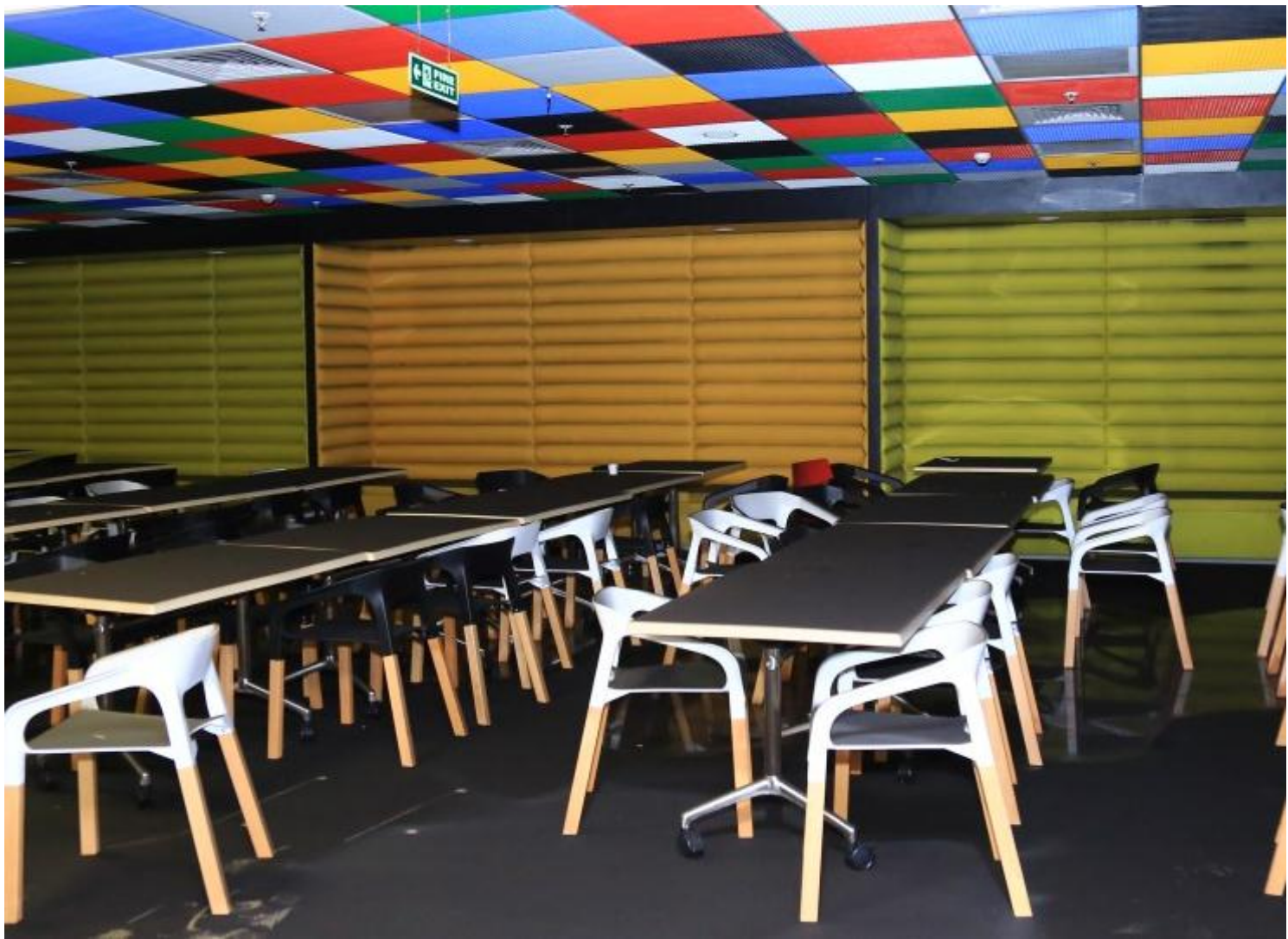
Soot seen on horizontal surfaces delivered through HVAC ducts and ceiling diffusers
