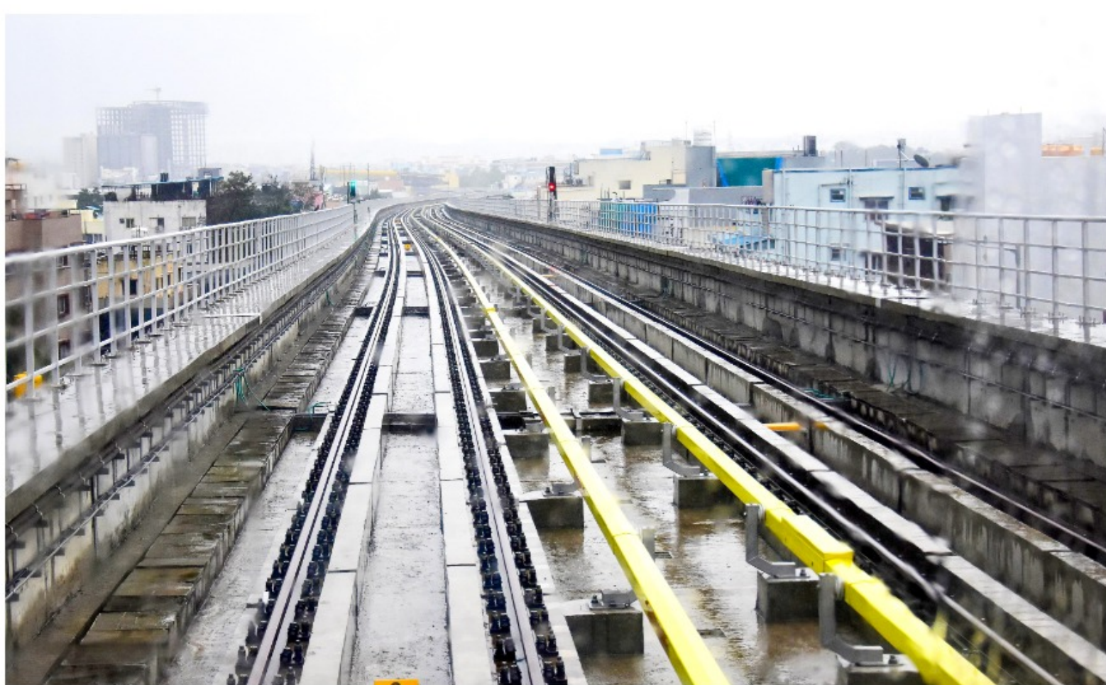
A close-up view of the tracks of the Yellow Line Metro (File Photo: IANS)
